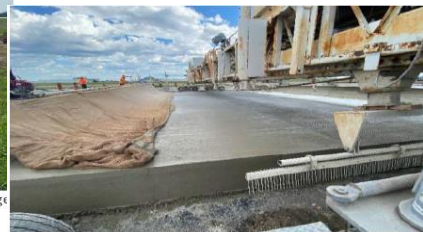
Stage 1D: Burlap, tining and white cure finishing of PCC slip form paving.
