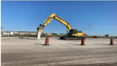
Stage 2A: Breaking existing concrete slabs on Runway keel section at Taxiway D5 intersection for removal.
