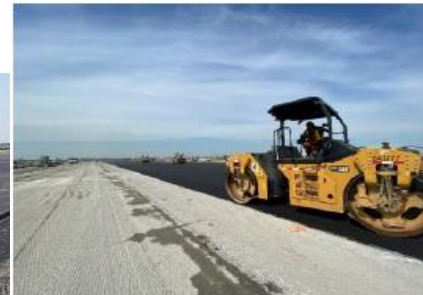
Stage 1C: Rolling and compaction of base asphalt on runway keel section.
