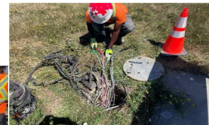
Stage 1C: Re-connect the cables from north runway side Taxiway D3 stop bar to the transformers in the pull pit
