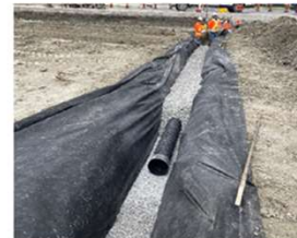
Stage 1A: Installation of 250mm dia. subdrain placement at Taxiway D8 centerline.
